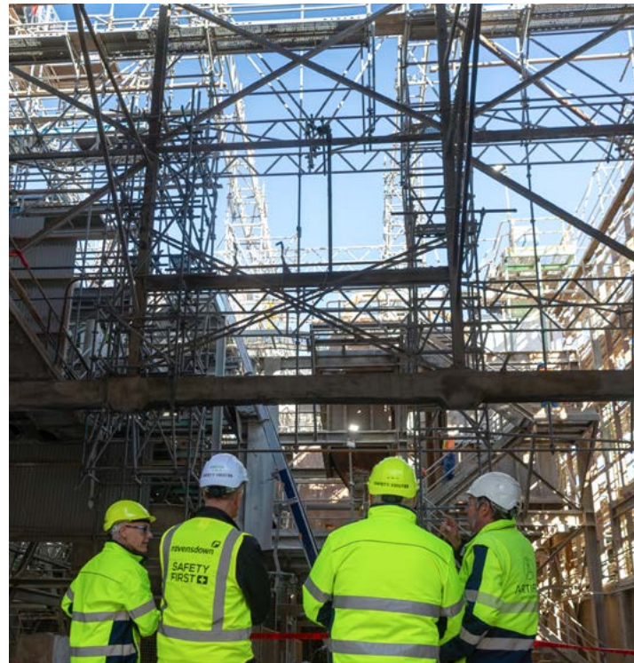
< Tonnes of scaffolding safely supported the construction of a new roof for the manufacturing plant at Napier Works.
