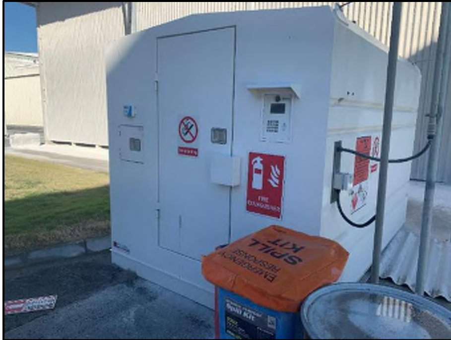
Photograph 25: View of the Diesel AST to the East of No 2 Despatch
