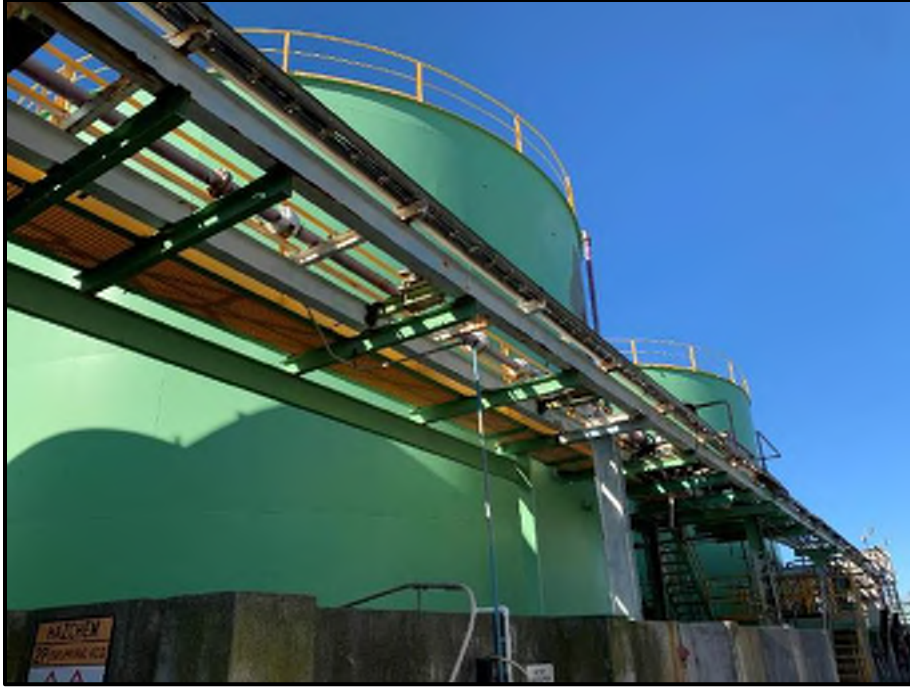
Photograph 15: General View of the Bunded Acid Tanks on Part Section 32 Block I Clive SD
