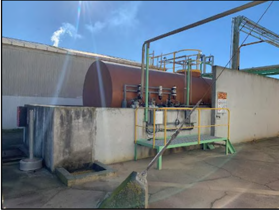
Photograph 13: General View of the Bunded Diesel Tank on Part Section 32 Block I Clive SD
