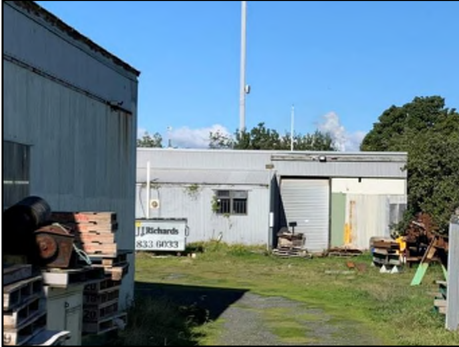
Photograph 5: General View of the Old Refrigerator Store to the Rear of the Above Engineering Workshop
