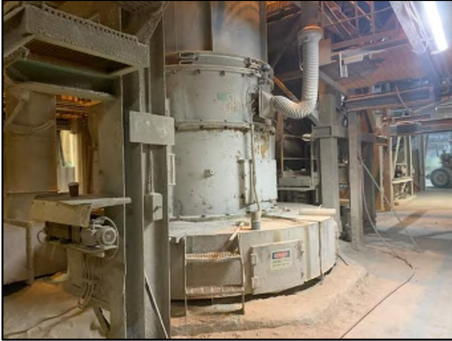
Photograph 23: View of Grinding Mill Equipment Inside the Manufacturing and Granulation Building
