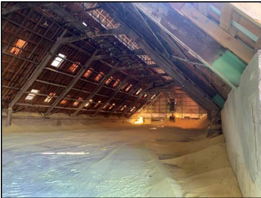
Photograph 34: Internal View within the Older Sulphur Store Towards the South of the Site
