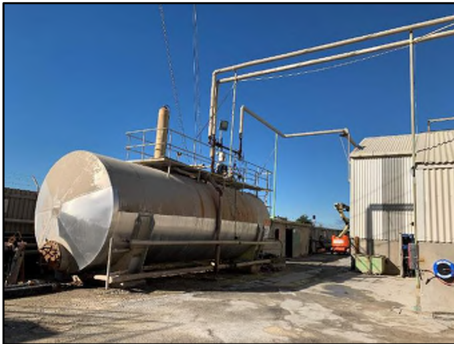
Photograph 26: View of the Molten Sulphur AST South-East of the Manufacturing and Granulation Building
