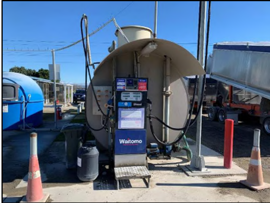
Photograph 19: View of the ASTs at the Truck Depot in the North of the Site
