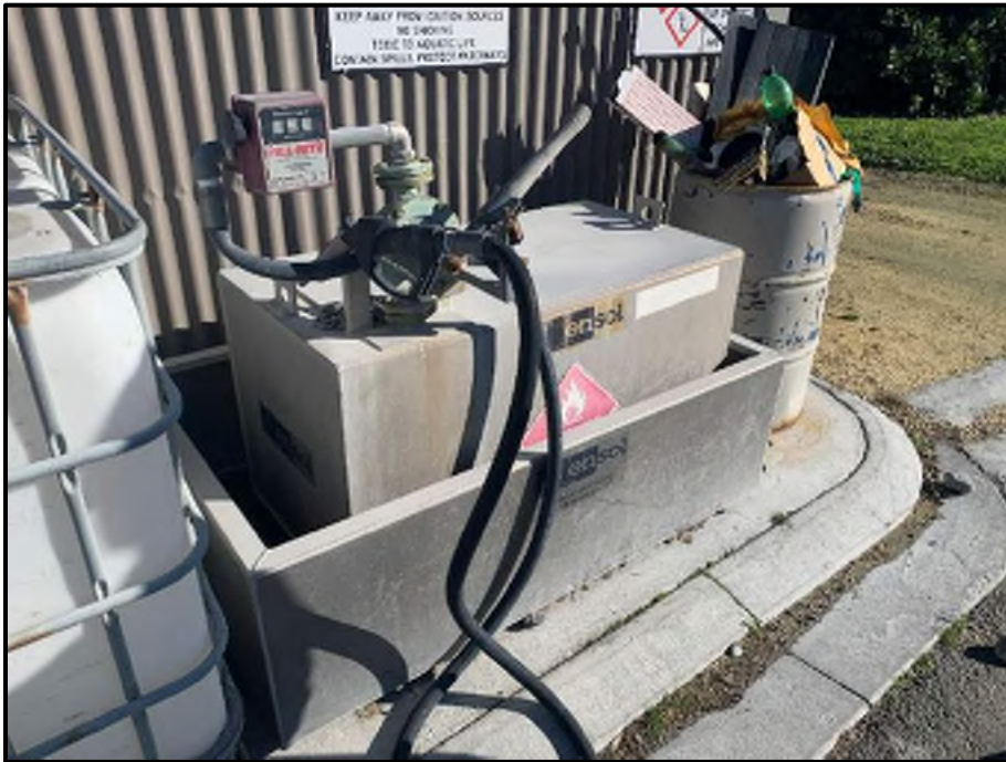
Photograph 22: View of the c.500 litre Petrol AST in the North of the Site
