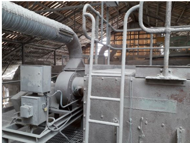
Photo 4 Cloth Filter Baghouse
