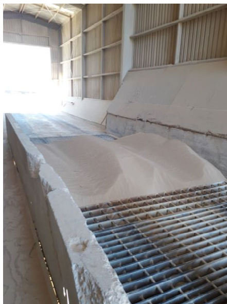
Photo 1 Truck Unloading Hopper
