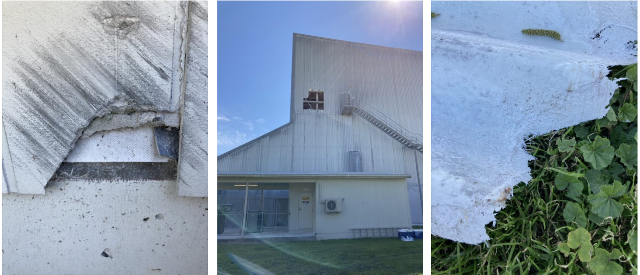
Figure 8: Deterioration of suspected ACM building materials near TP101 in the northern part of the site.
